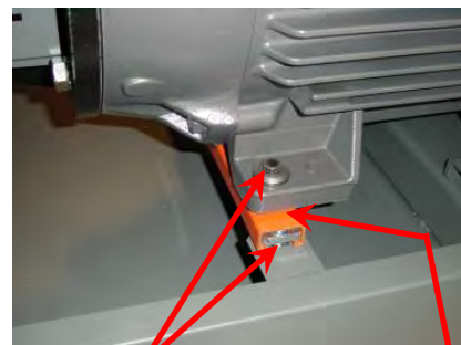
Motor Cleat from the Rear of Unit.
