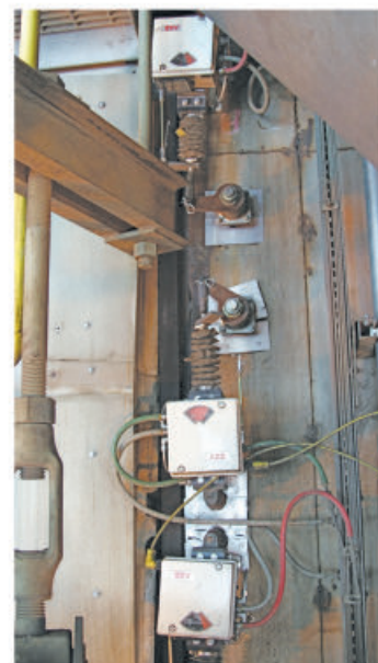
LP20 Pneumatic Linear Actuators with AV Positioners Installed on Windbox Dampers
