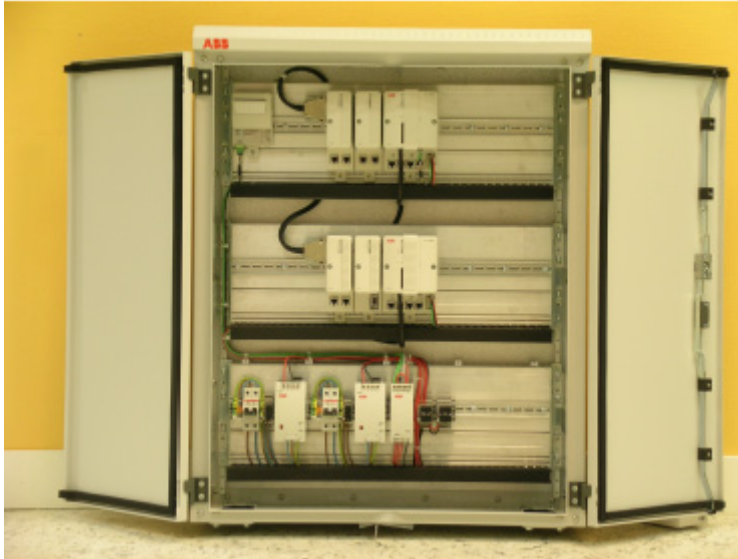
Figure 49. Cabinet with Controller on prefabricated aluminium profiles
